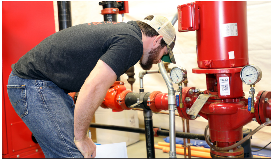
Hands-on training includes capturing the discharge pressure of a fire pump during an annual flow test.
